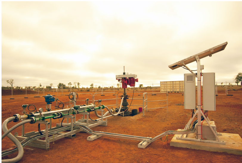
Oil field pump station
